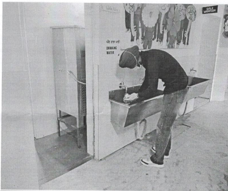
After RO (Water Cooler Tap- Near Class Room XIIE)
